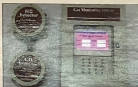
Toxic and Combustible Gas Monitoring System
